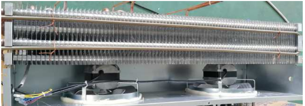
Defrosting heater view:
